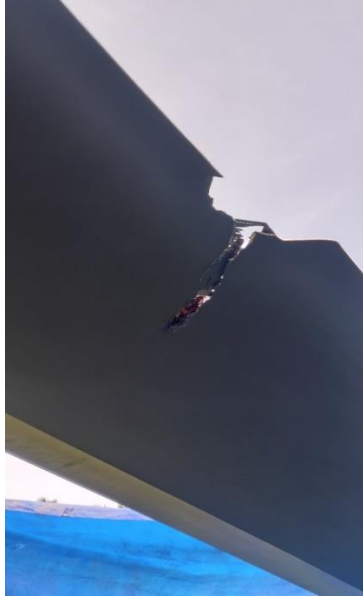
(Fig. 16: Main Rotor Blade s/n-AW1812 found cracked near Trim Tab)
